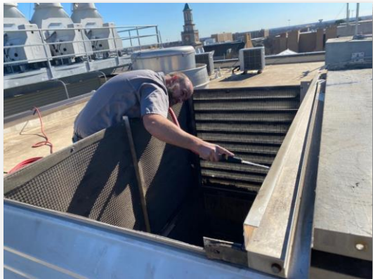
Matt cleaning air intake on the roof of Life Science.
