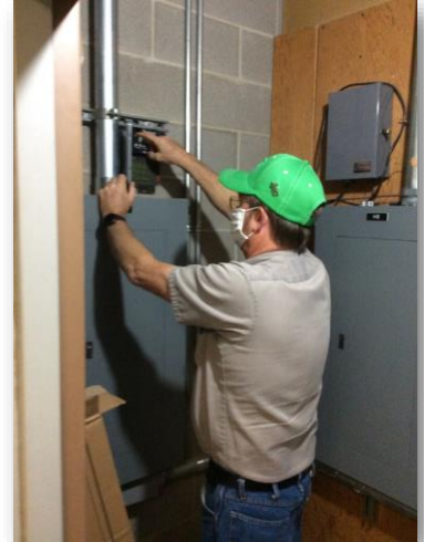
Roger in our electric shop resetting the time clocks that bring on outside lighting.
