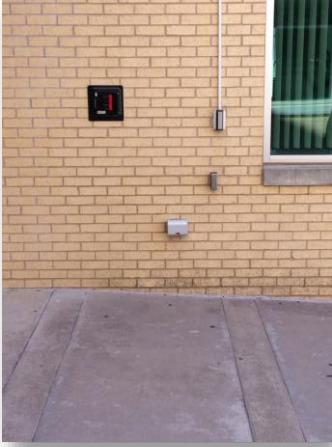
GFCI plug that the Electrical group is installing around campus for a student project to monitor air quality.
