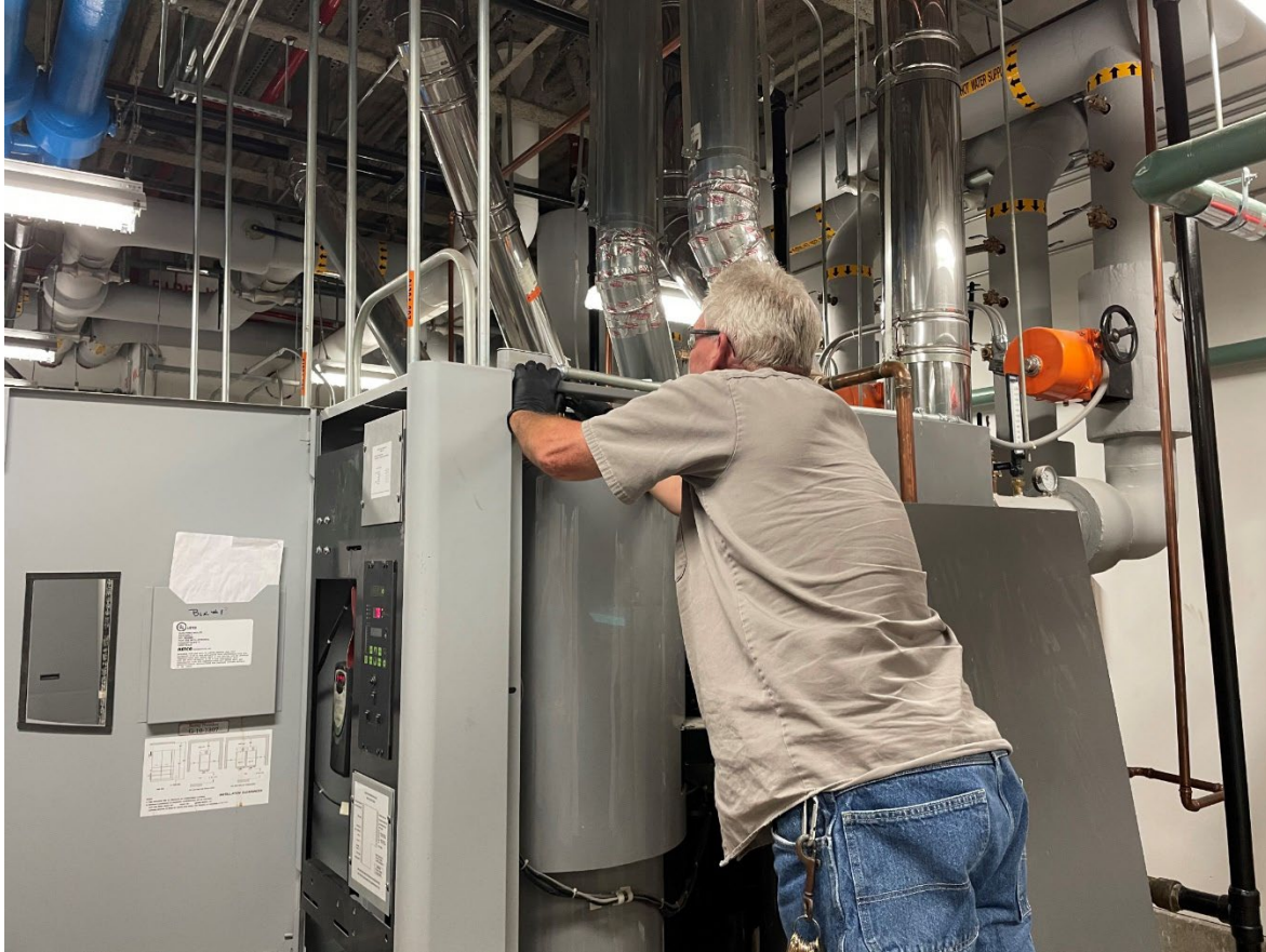
Bruce doing PMs on our boilers
